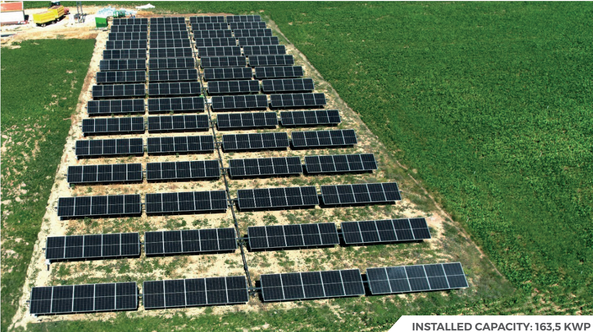
INSTALLED CAPACITY: 163,5 KWP
